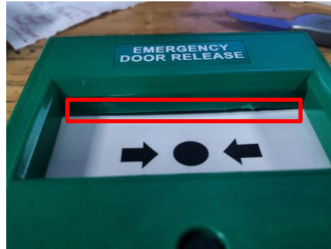
Activated – note flex in plate and gap
